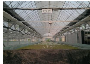
Smart LED Lighting system
